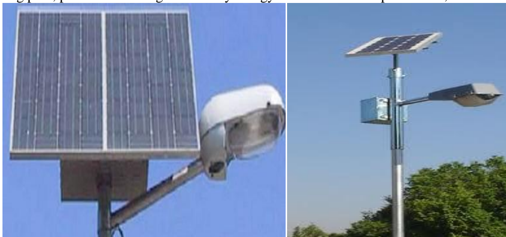
Figure.2. Solar PV System installed on Mall Road,Peshawar,Courtesy of Cantonment Board Peshawar
